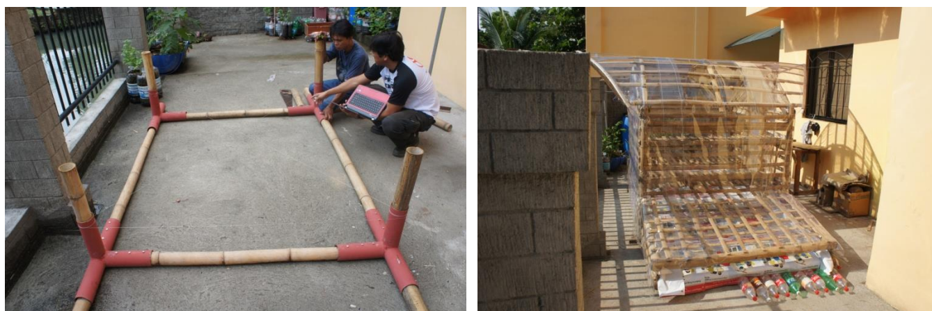
Figure 11. Top left photo: the author (in white shirt) as he was giving instructions to the carpenter. Notice the metal joints for the bamboo poles. Top right photo: the bamboo dryer as it was built.
